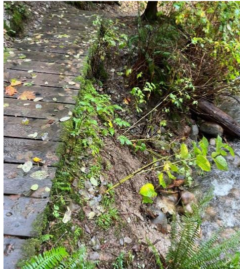
Photo 10. Bank erosion under cutting Boardwalk.
