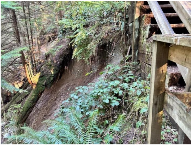
Photo 7. Bank erosion undercutting stair footings.
