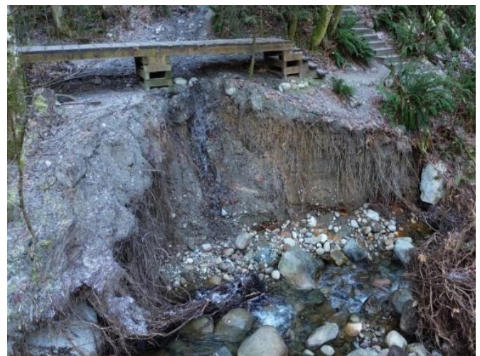
Photo 4. Bank erosion under cutting boardwalk footings.
