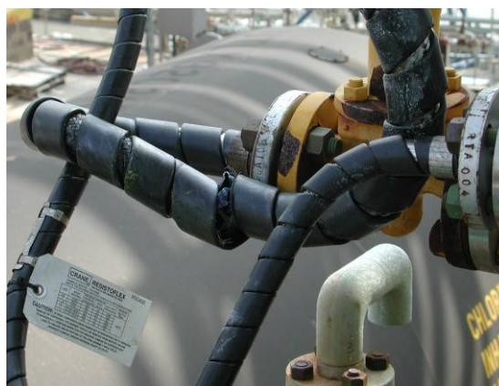
Figure 2. Honeywell ruptured chlorine transfer hose
