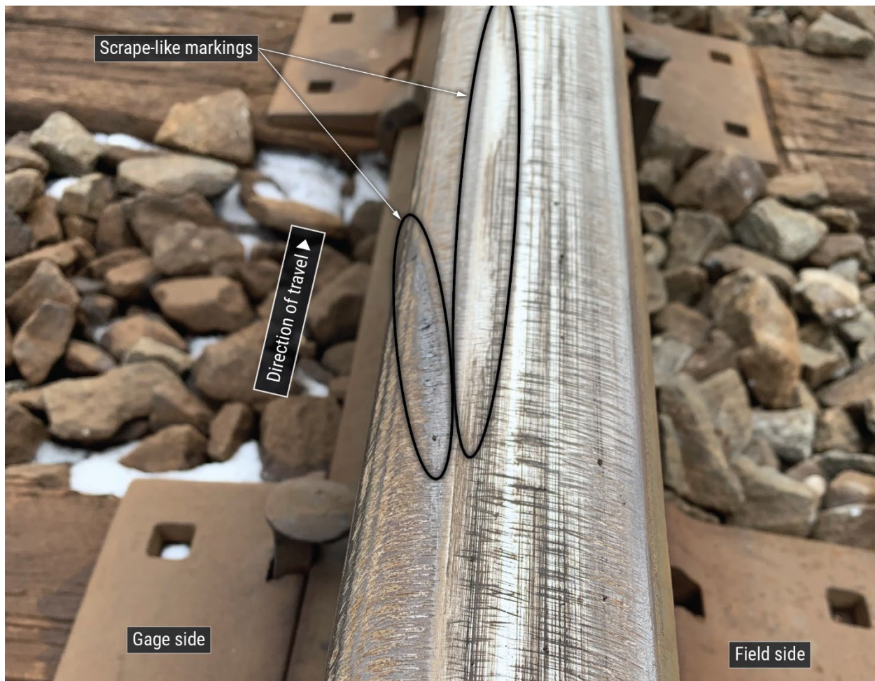
Figure 11. South running rail at MP 49.5.
