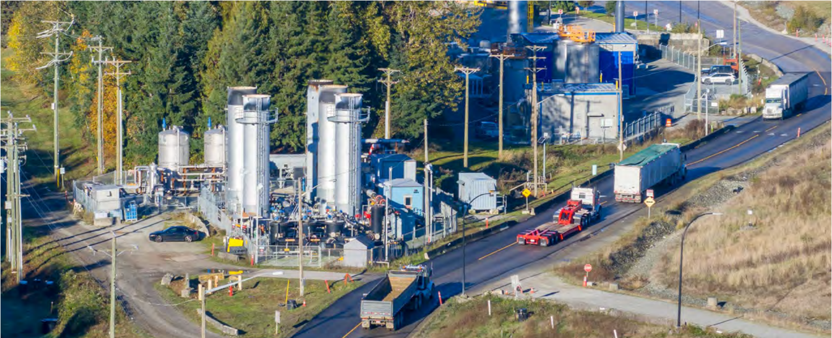
Vancouver Landfill flare station
