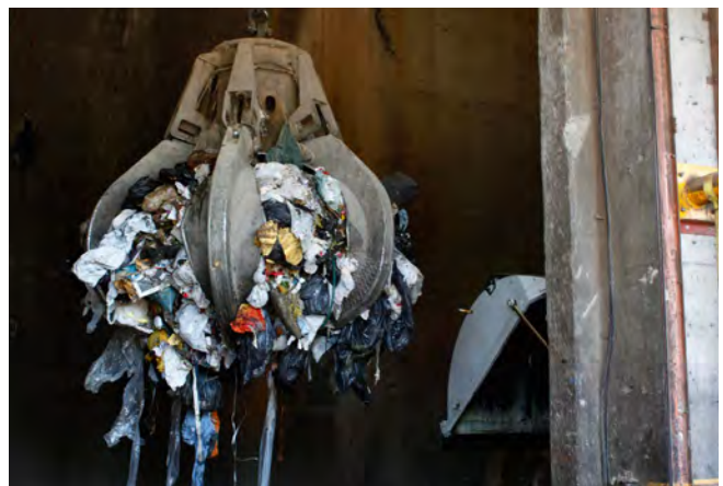
Garbage claw at the Waste-to-Energy Facility
