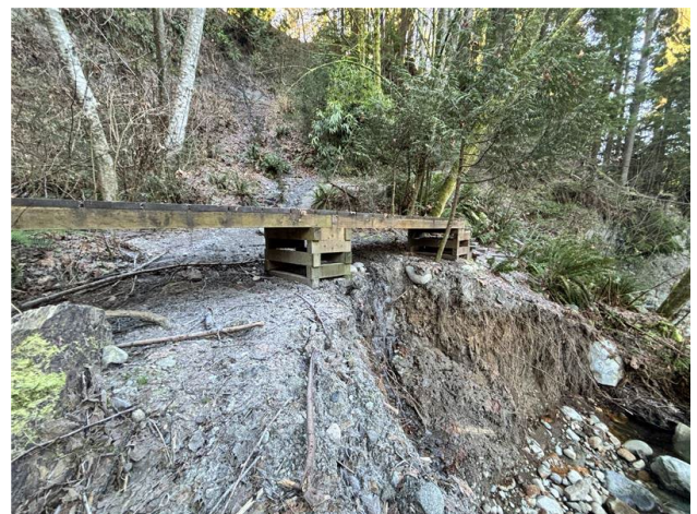
Photo 4. Bank erosion under cutting boardwalk footings.
