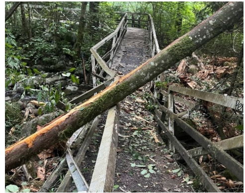
Photo 2. Damaged southern bridge.
