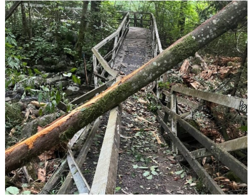
Photo 2. Damaged southern bridge.
