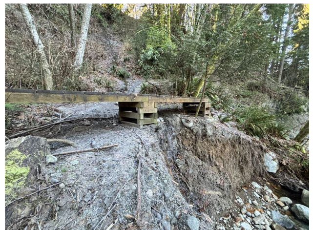
Photo 4. Bank erosion under cutting boardwalk footings.
