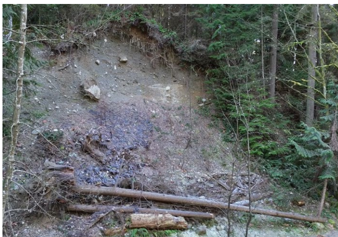
Photo 5. Large landslide area directly above trail. Large rocks regularly roll down onto the trail.
