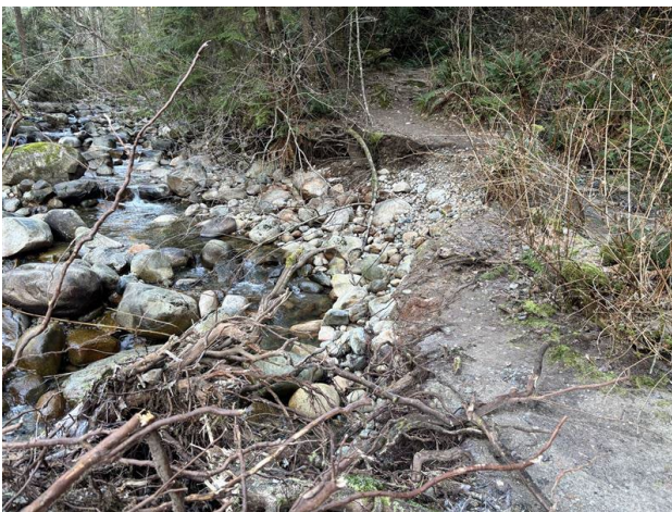
Photo 3. Trail fully washed away.
