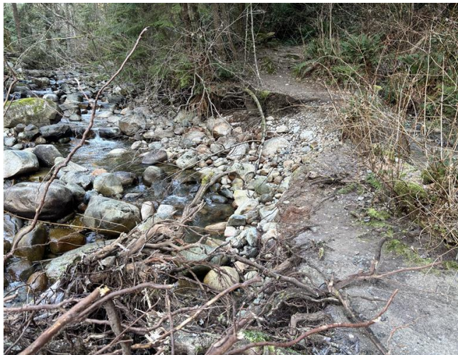
Photo 3. Trail washed away from creek erosion.
