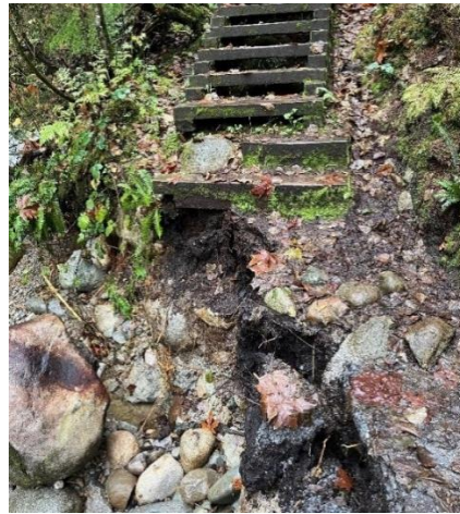
Photo 8. Erosion undercutting stairs.
