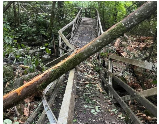
Photo 2. Damaged southern bridge from tree failure.
