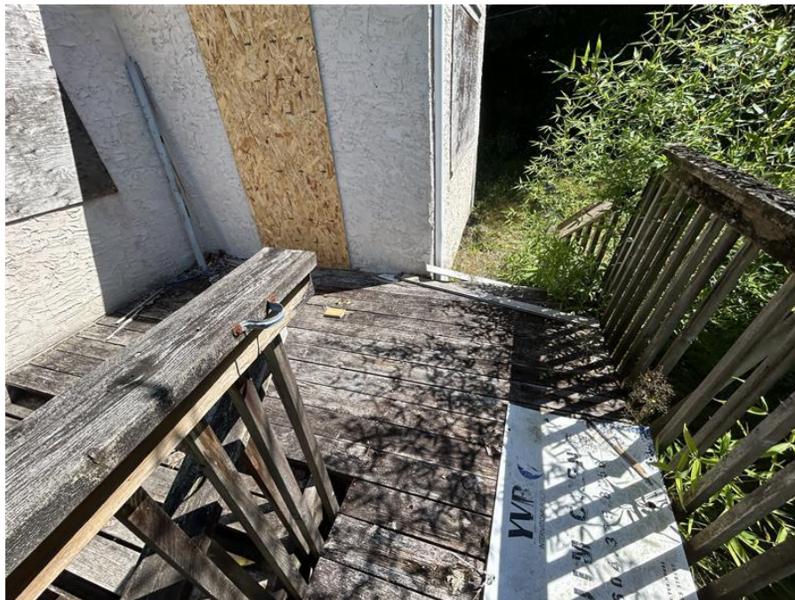
View of front entrance and patio/porch to house, accumulated materials and growths in front yard:
