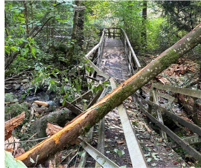
Fallen tree damage to southern bridge
