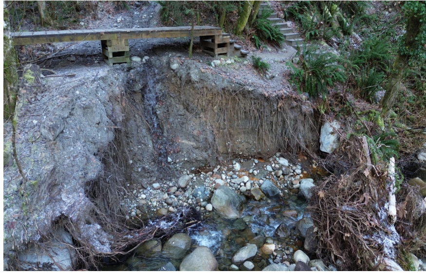
Bank erosion under boardwalk (glacial till exposure)
